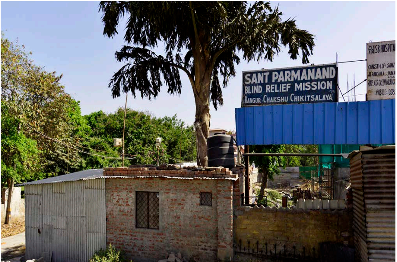
This building is coming up right now on the Yamuna floodplain near Nigambodh Ghat. The builders say it will be a ten-storey charitable eye hospital. There are conflicting claims on whether the Delhi Development Authority or anyone else in a position of power has given permission
