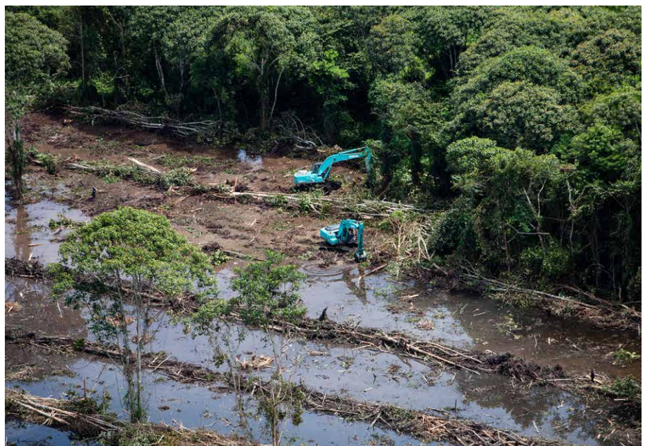
Excavators clear carbon-rich peatland forest in an oil palm concession, Central Kalimantan, Indonesia (Image © Kemal Jufri / Greenpeace)
